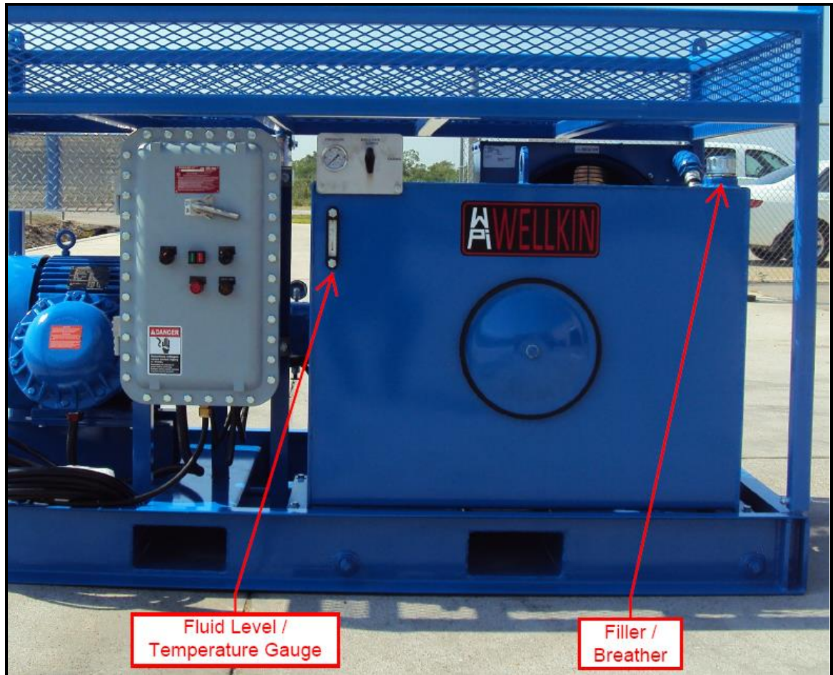
Figure 2: Tank Level Gauge and Fill Location
