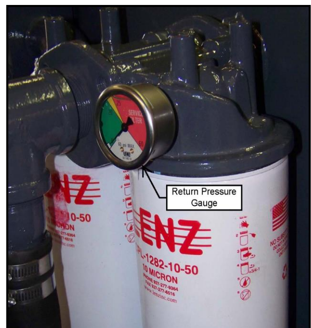
Figure 8: Return Pressure Gauge
