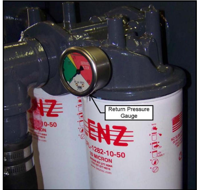
Figure 8: Return Pressure Gauge
