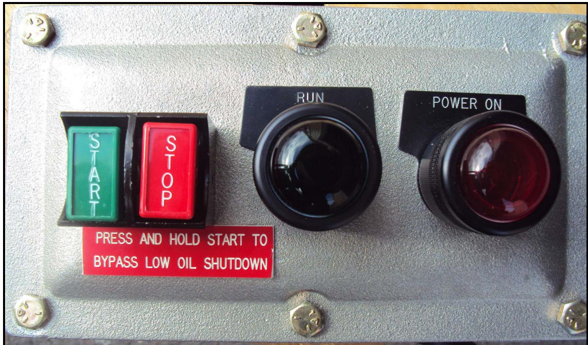
Figure 6: Remote Start/Stop Panel
