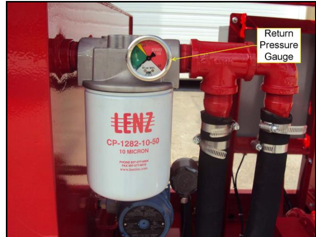
Figure 6: Return Filter Pressure Gauge
