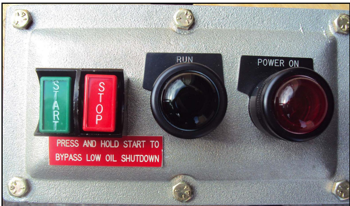
Figure 7: Remote Start/Stop Panel
