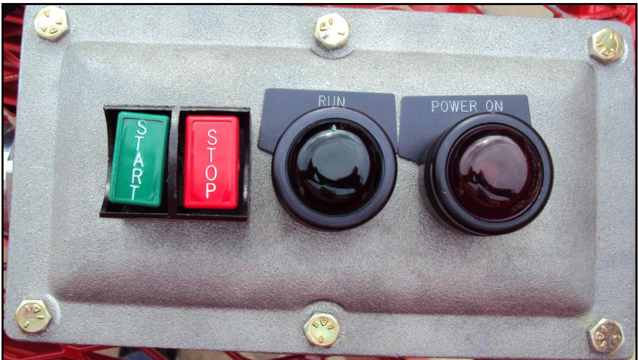
Figure 7: Remote Start/Stop Panel
