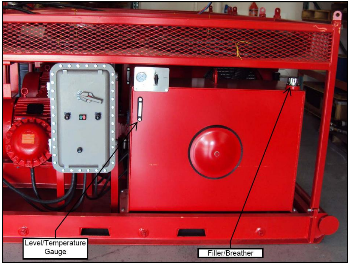
Figure 2: Tank Level Gauge and Fill Location
