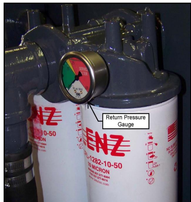
Figure 8: Return Pressure Gauge
